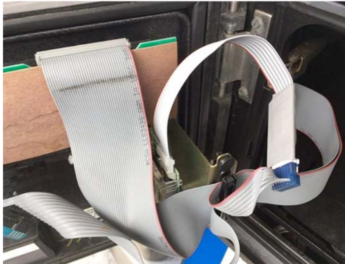
FIG. 8 A Bluetooth Custom Skimmer Secreted Inside a Gas Pump
