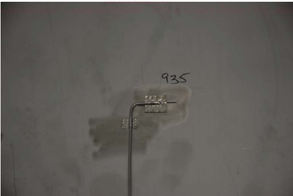
FIG. 3 Photo of Typical TC Installation
