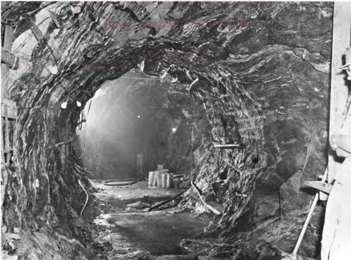
FIG. 4 View of Final Radial Jacking Test Chamber Excavation and After Installation of Extensometers (1) Courtesy of the US Bureau of Reclamation
