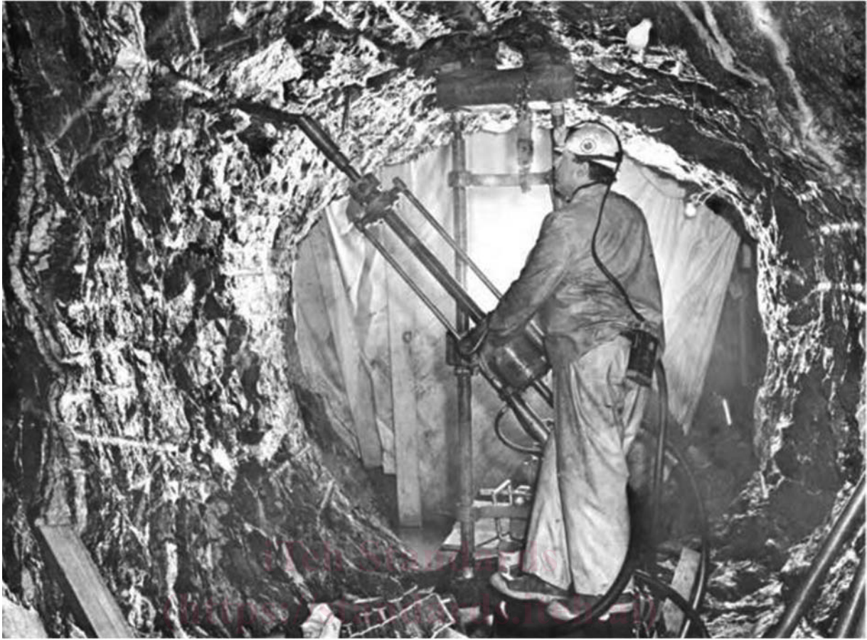
FIG. 5 Drilling Instrumentation Holes for Radial Jacking Test (1) Courtesy of US Bureau of Reclamation
