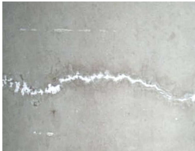
FIG. 3 Calcium Carbonate Filled Crack
