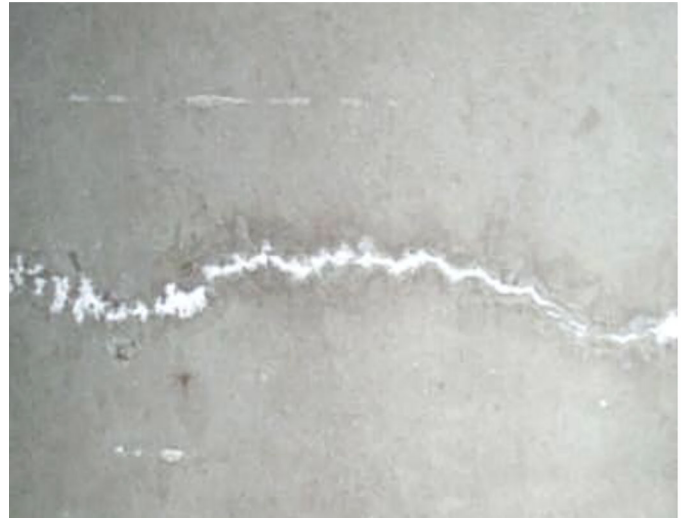
FIG. 3 Calcium Carbonate Filled Crack
