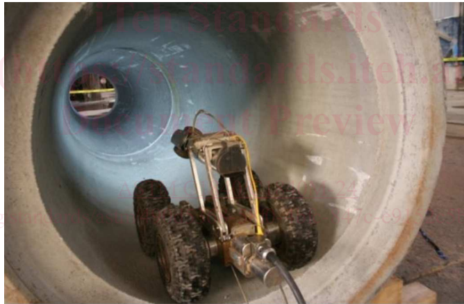
FIG. 2 Remote Inspection Camera
