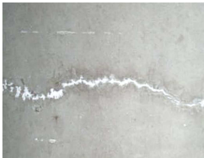
FIG. 3 Calcium Carbonate Filled Crack
