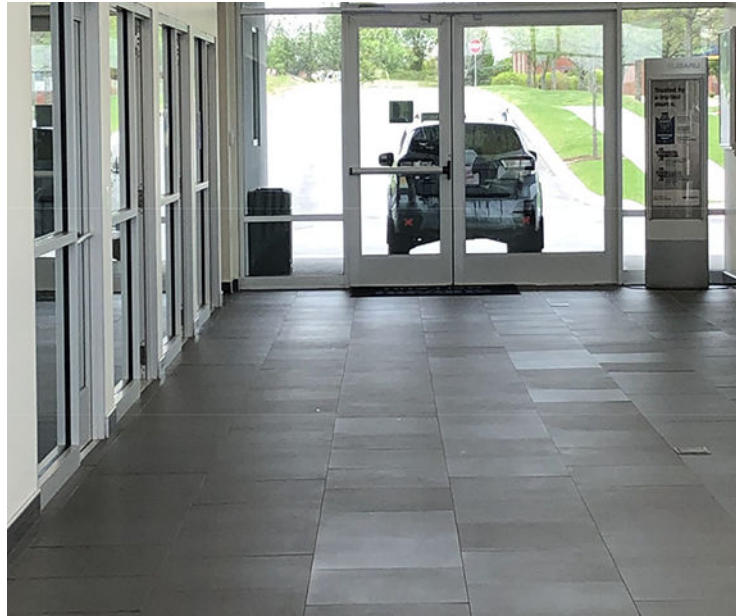
FIG. 1 Low Angle Light Defect Visible in an Installation
