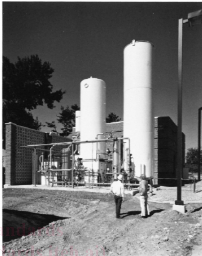
FIG. 1 High-volume Oxygen Users Buy the Gas in Bulk, Storing It in an Adjacent Facility
