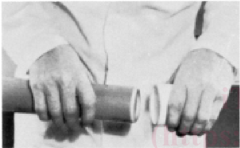
FIG. 7 Pipe Entering Dry Fitting
