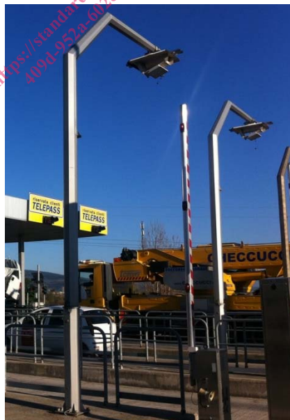
Figure 3: Typical HDR-DSRC RSU installation
