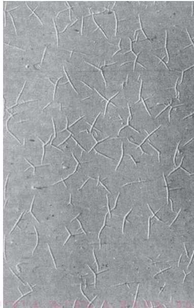
Figure 5 — Crow's foot cracking
