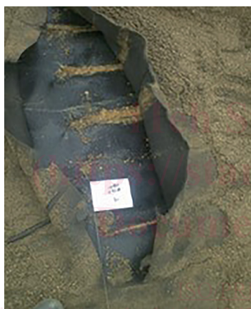
Figure 3 — Barrier damage due to construction traffic
