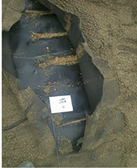
Figure 3 — Barrier damage due to construction traffic
