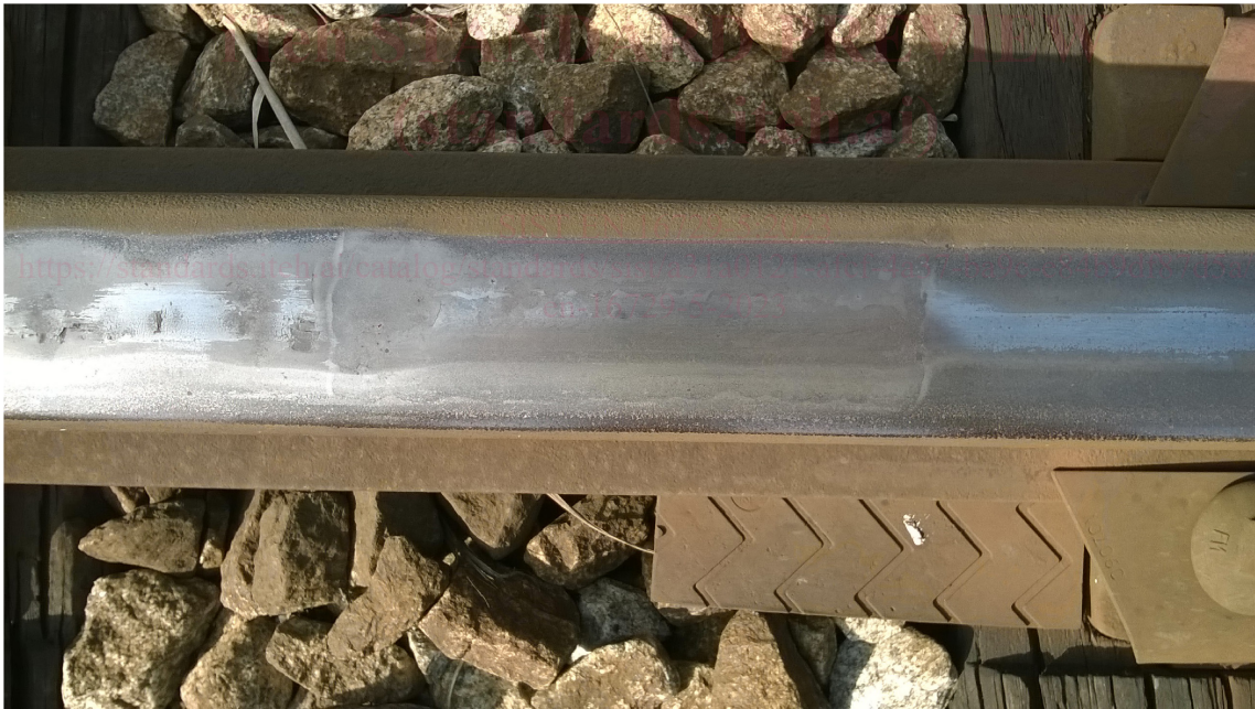
Figure 1 — Porosity on electric arc repair welds (a)
