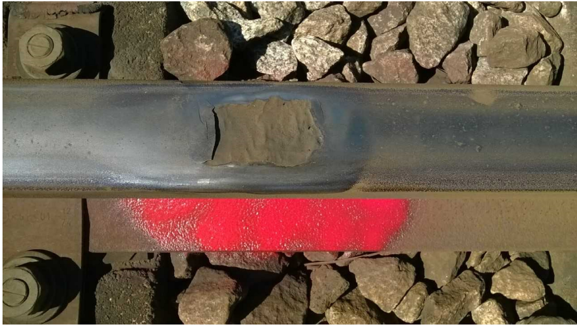
Figure 5 — Lack of fusion
