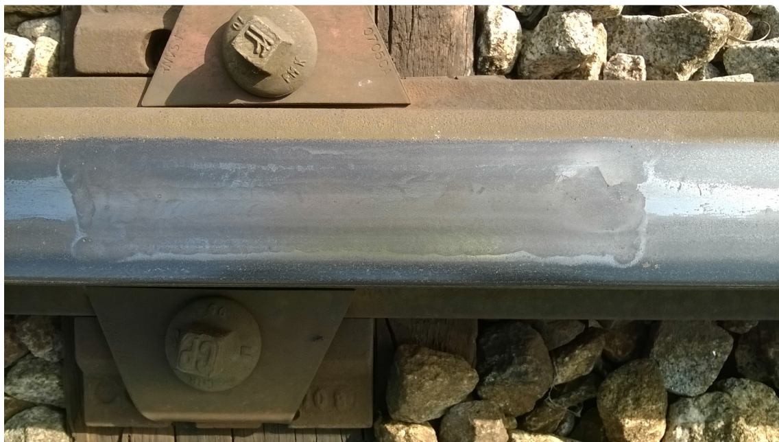
Figure 2 — Porosity on electric arc repair welds (b)
