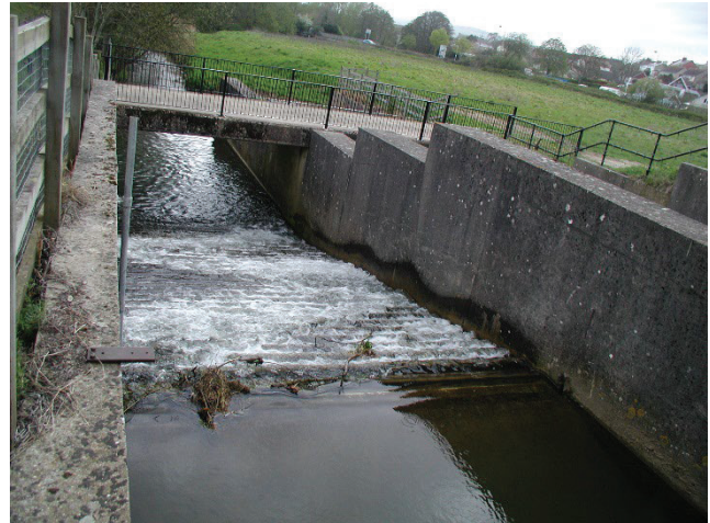
b) Baffles in operation before maintenance has been carried out (viewed from upstream)
