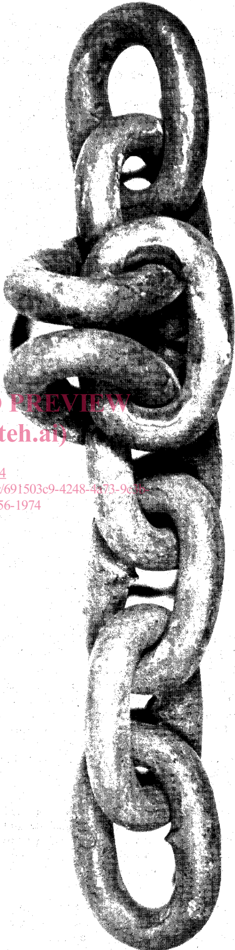
FIGURE 7 – Visual inspection for wear
