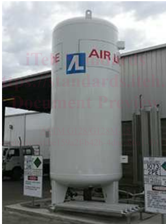
FIG. 2 Cryogenic Oxygen Storage Image courtesy of Air Liquide America
