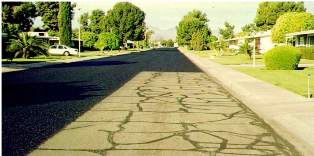
FIG. X1.1 Example of Block Cracking Due to Aging
