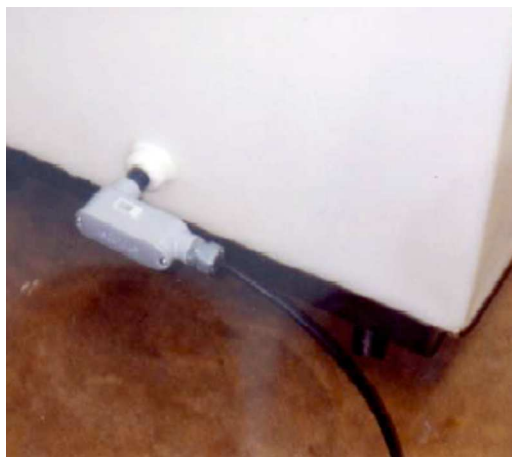
FIG. 6 Heater Conduit Boc Installed on Tank
