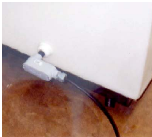
FIG. 6 Heater Conduit Boc Installed on Tank
