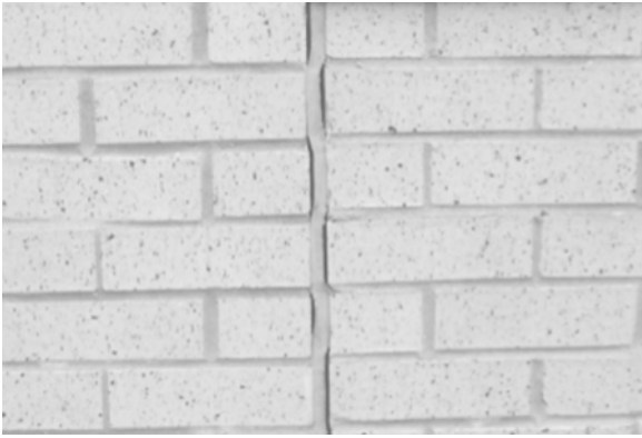
adhesion failure, n—in building construction , failure of the bond between a sealant and a substrate.
